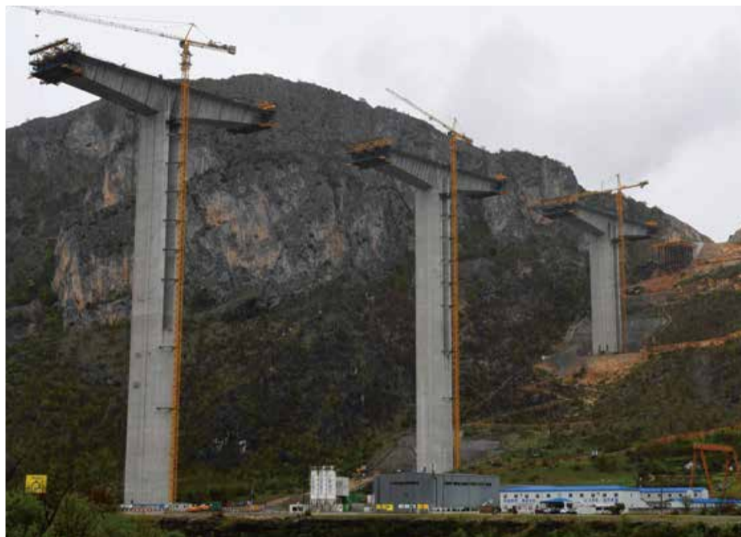
The bridge section of a highway connecting the city of Bar on Montenegro's Adriatic coast to landlocked neighbor Serbia, near the village of Bioce, north of Montenegrin capital Podgorica, which is being constructed by China Road and Bridge Corporation (CRBC), the large state-owned Chinese company, April 8, 2019.
